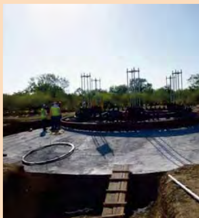
Ventika Wind Farm
